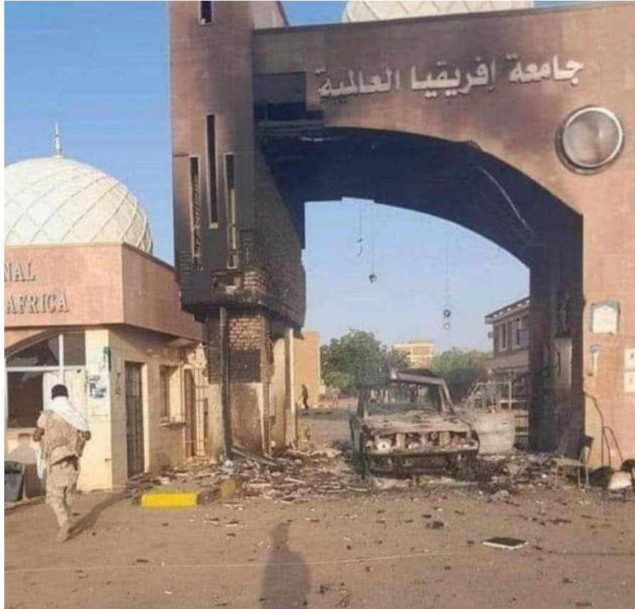
Figure 2: International University of Africa; showing an example of the destruction to infrastructures to medical schools in Khartoum state. Also in the picture, a member and a bomb shelled vehicle of RSF as they used the campus as a militia base.
